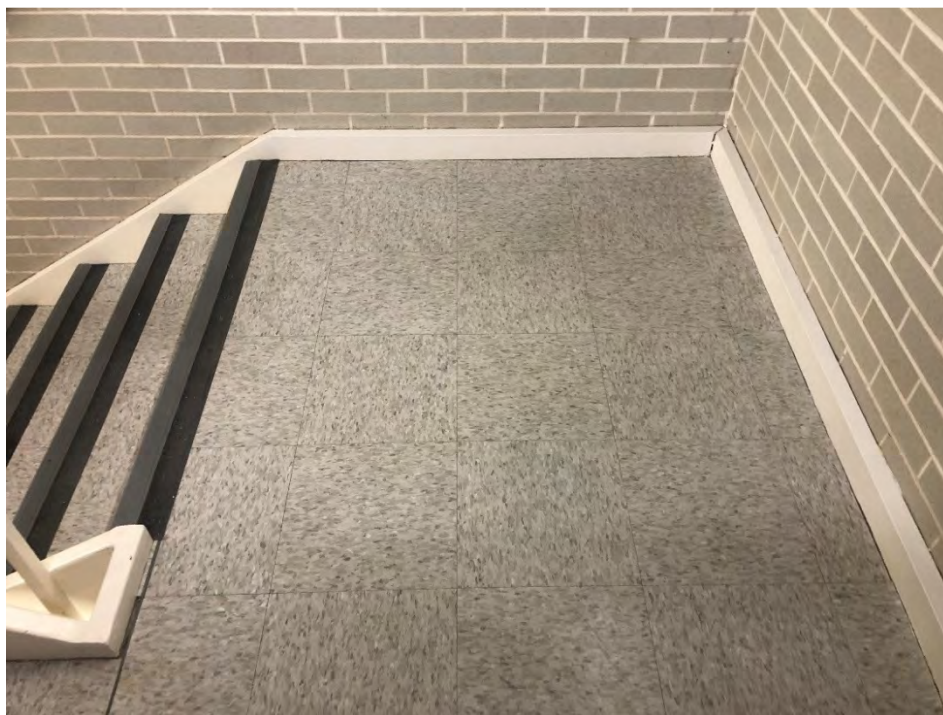
Photograph 9: Black mastic associated with white with gray streaks 12x12" floor tile, observed in the Tower. Sample number 74-B.
