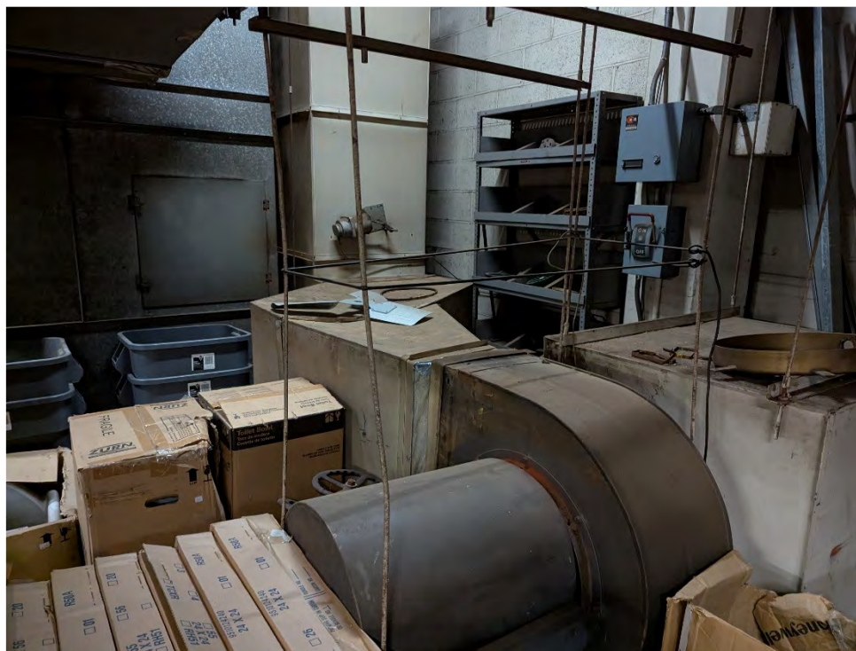
Photograph 11: White duct vibration dampener, observed in the Tower. Sample number 109.
