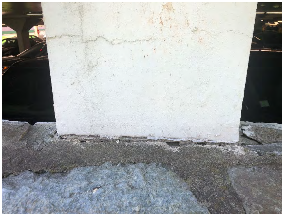
Photograph 22: Sealant between stone and column, observed in the Tower garage. Sample number 110.
