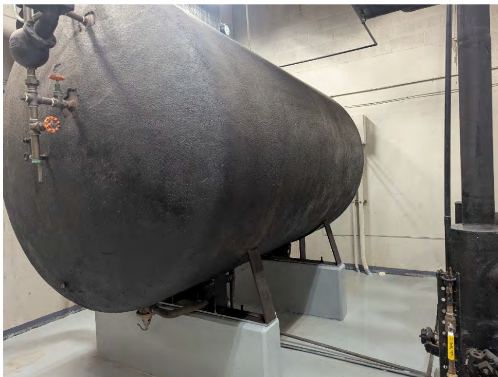
Photograph 19: Tar coating on large black water heater, observed in the Tower. Sample number 11.
