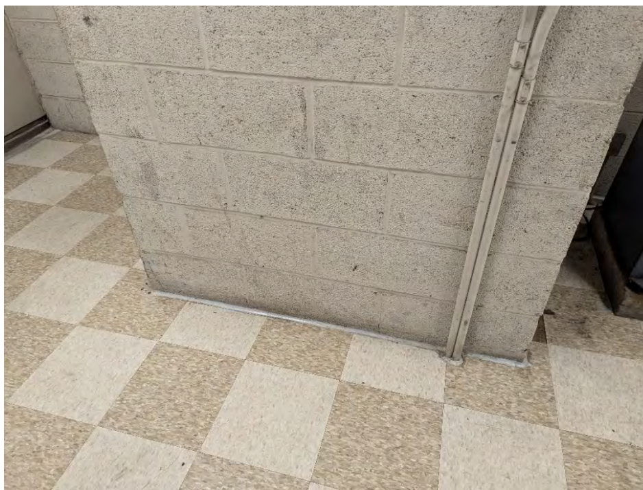
Photograph 10: Mastic associated with white with tan streaks 12x12" floor tile and tan with white streaks 12x12" floor tile, observed in the Tower. Sample numbers 86-B and 88-B.
