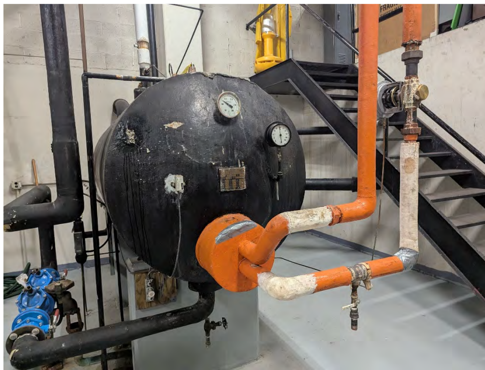
Photograph 18: Insulation and canvas on small black water heater, observed in the Tower. Sample number 8.
